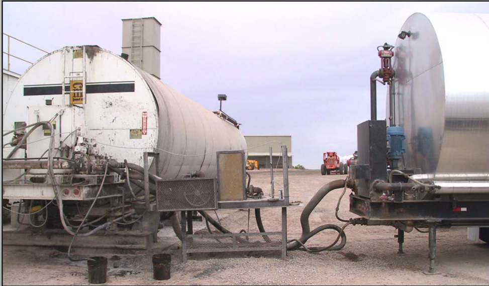
Binder Supply Line Connects Directly To Hot Mix Plant, Completely Bypassing Their Tank and Pump
